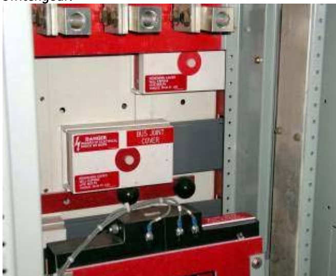
Figure 4: Low voltage insulated/isolated bus in a rear access Powerbreak II switchboard or AKD-10 or Entellisys switchgear.
