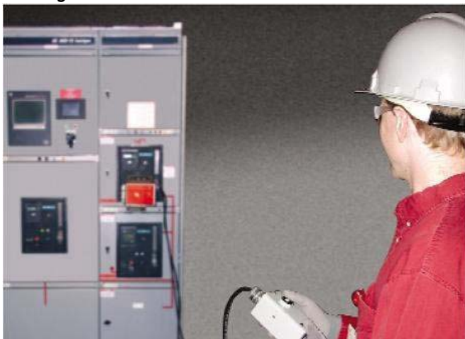
Figure 2: Using a remote racking device on Wavepro low voltage power circuit breakers in AKD-10 switchgear.
